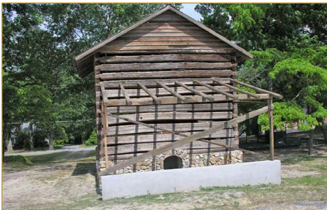
The barn sports the framework for the shelter. The gable ends are now complete and the entire structure awaits chinking next.
